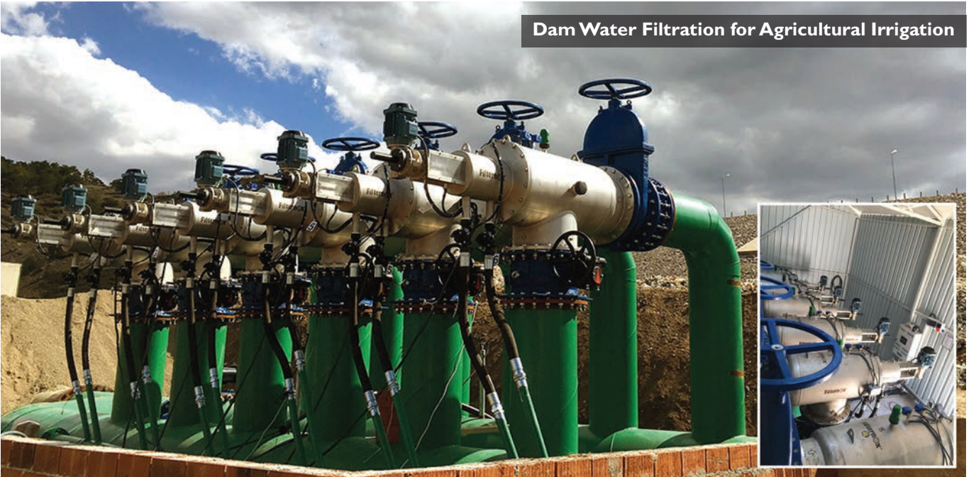
Two Stage Filtration of River Water for Drip Irrigation
