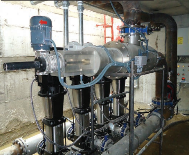
Water Filtration for Golf Course Irrigation
