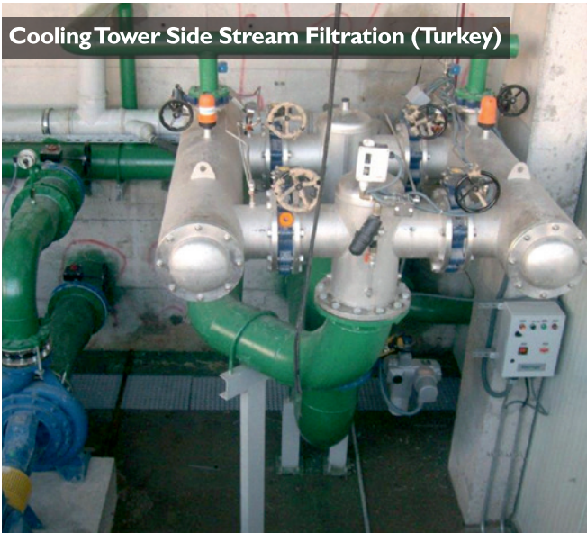
Cooling Tower Side Stream Filtration (Turkey)
