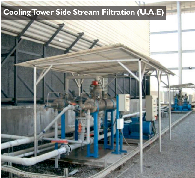
Plastic Industry, Cooling Water Filtration for Extrusion & Extruder (Turkey)
