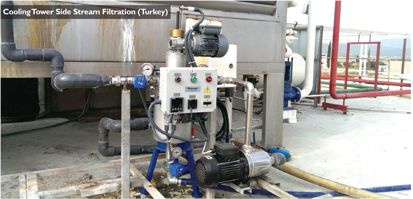
Cooling Tower Side Stream Filtration (Turkey)
