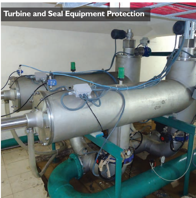
Turbine and Seal Equipment Protection
