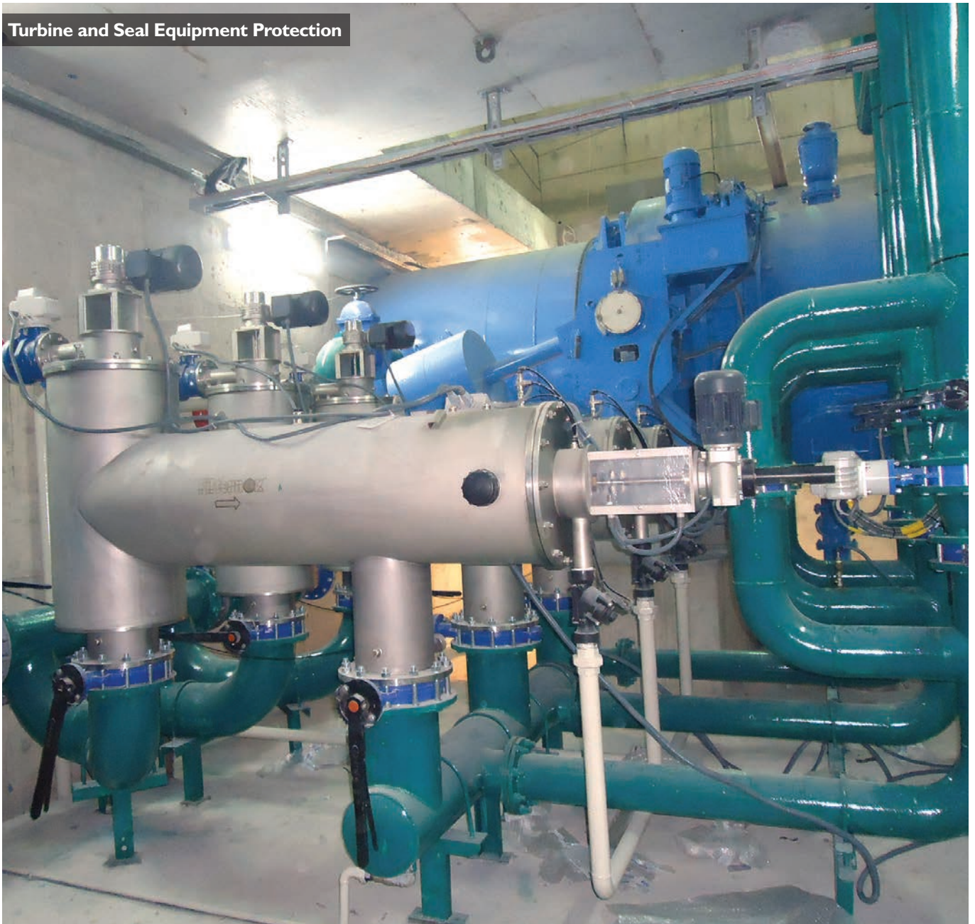
Turbine and Seal Equipment Protection
