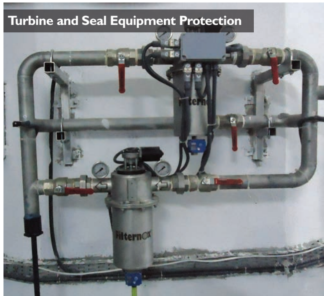
Turbine and Seal Equipment Protection
